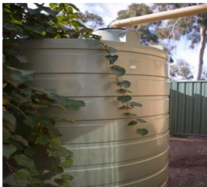
Rainwater tank (M. McAulay & DEWHA).
